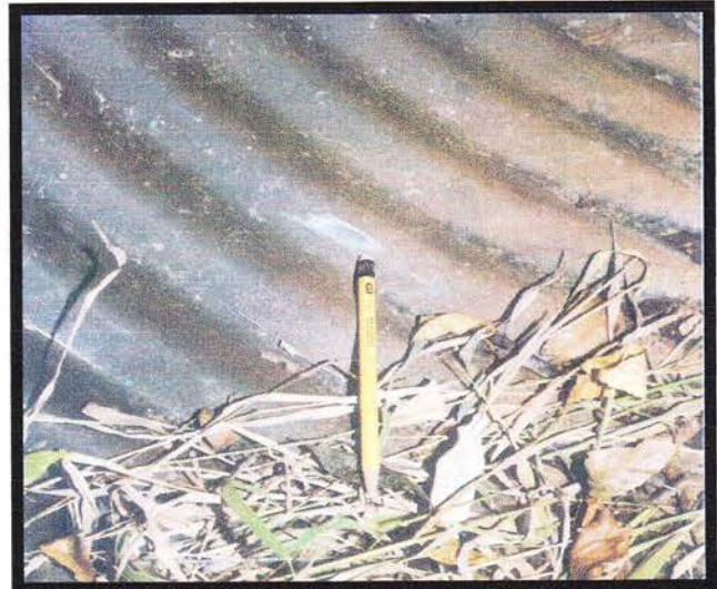
This 30" diameter, 3 mil polymer coated corrugated steel pipe storm drain has been subjected to acidic soil and conductive swamp drainage for ten years. As can be seen, the pipe is in "like-new" condition.
